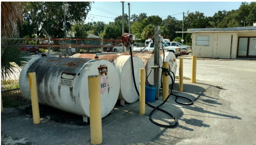
Neither spillage nor staining were evident beneath the above ground petroleum storage tanks on the subject parcel.
