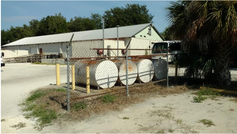
Four 500-gallon petroleum storage tanks on site. Two contain unleaded gasoline and two ASTs contain diesel fuel..
