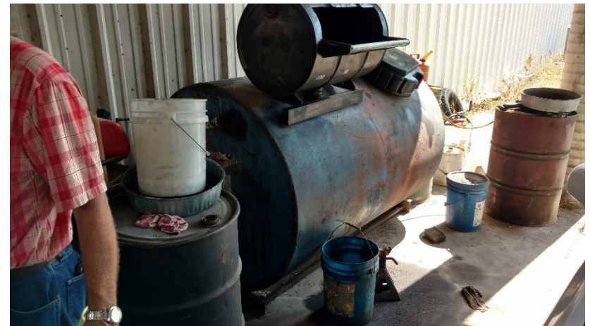
Waste oil receiving tank stored outside the bus repair garage. Oil staining is minimal and on a concrete pad. Waste oil is periodically pumped out and recycled by a local waste recycler.
