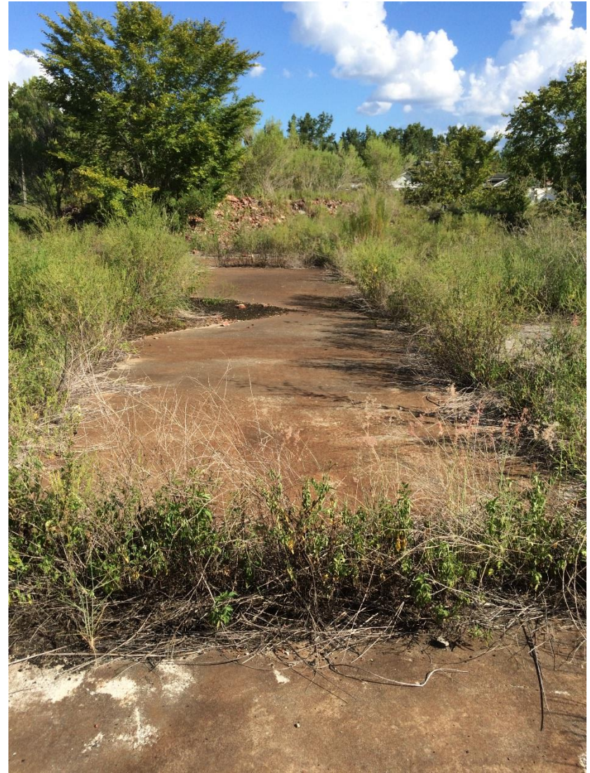
Concrete staining on various slabs in the rear yard.
