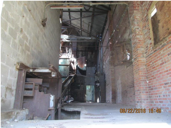
Boiler Room Interior.
