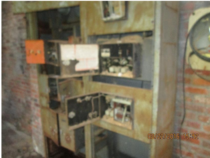
Electrical panel in the boiler room.
