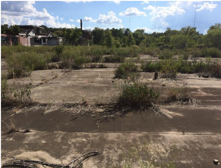
Concrete slabs from warehouse buildings.
