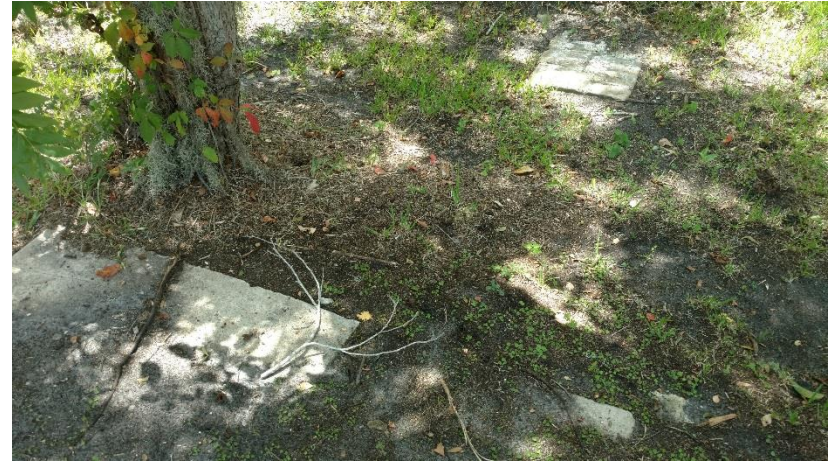
Old footings and concrete pads may have been used to support former ASTs.
