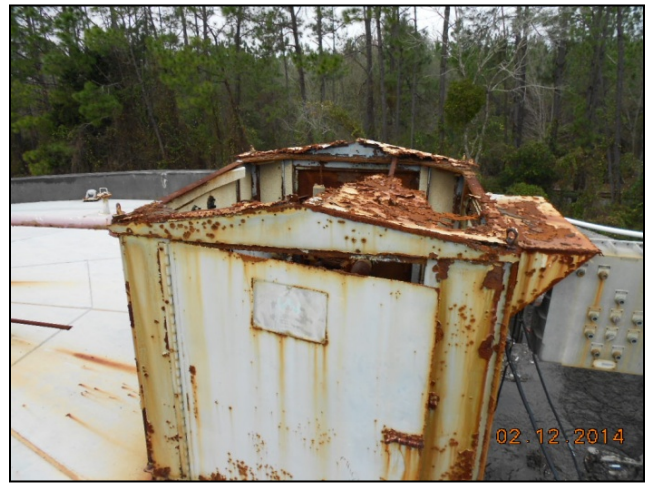
DIGESTER COVER / COMPRESSOR HOUSE
