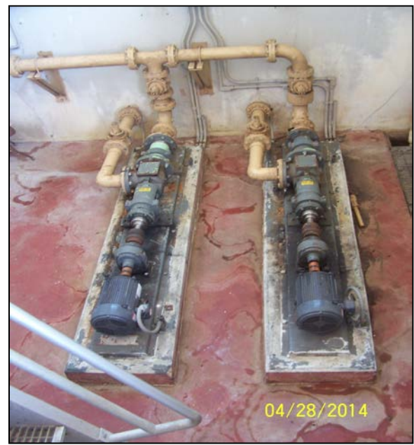
BELT-FILTER PRESS FEED PUMPS
