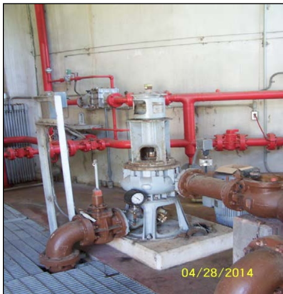
DIGESTER SLUDGE RECIRCULATION PUMP
