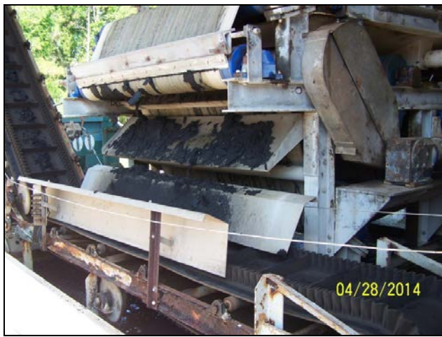
BELT-FILTER PRESS DEWATERED SLUDGE DISCHARGE TO CONVEYOR
