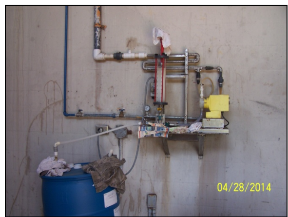
SLUDGE DEWATERING POLYMER FEED SYSTEM
