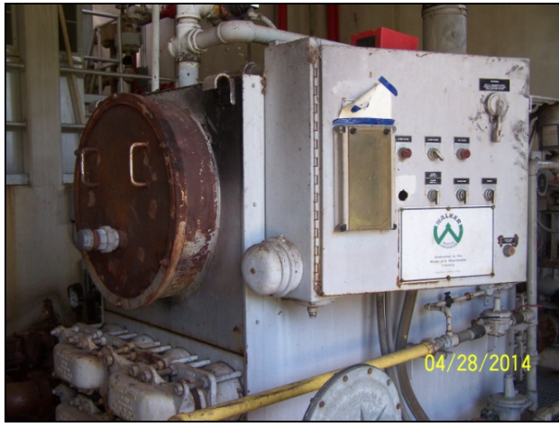
DIGESTER SLUDGE HEATER UNIT
