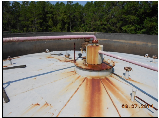
DIGESTER COVER / PIPING
