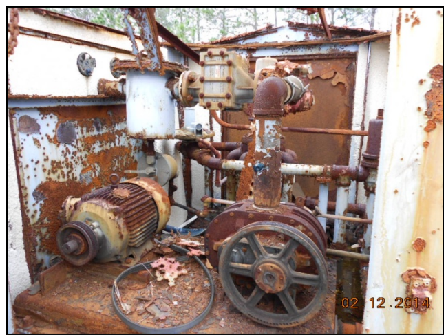
DIGESTER COMPRESSOR HOUSE (INTERIOR)
